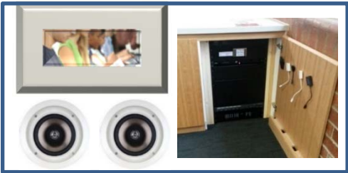
Classroom 4 All Equipment
