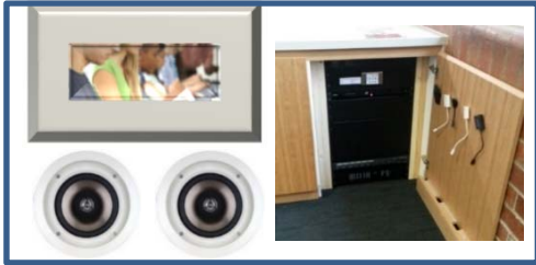
Classroom 3 All Equipment
