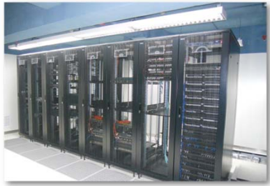
A dedicated data center or a functional area within
