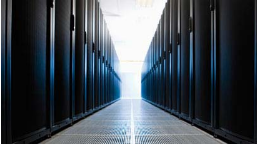
IT/Data Center Space
